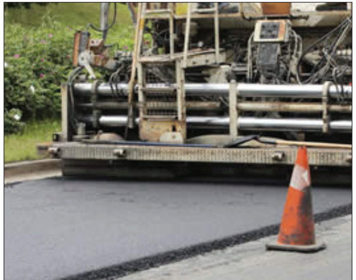
Thanks to a recently completed Street Index, the Streets and Stormwater Department is in a better position to prioritize street improvements.
